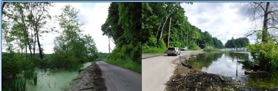
Debris and sediment on the road after 2017 flooding. Notice how close the water is to the road, with little soil left.
