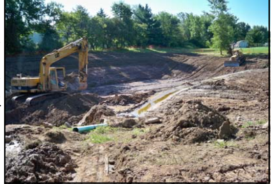
The much larger stormwater pond that will also provide stormwater treatment to the Ridge Meadows Subdivision.
