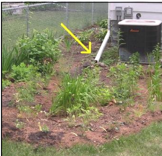
Downspout disconnect into rain garden. (Photo: commons.wikimedia.org)
