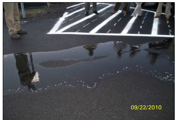
The water infiltrating through the porous pavement a few seconds after five gallons of water was poured on it.
